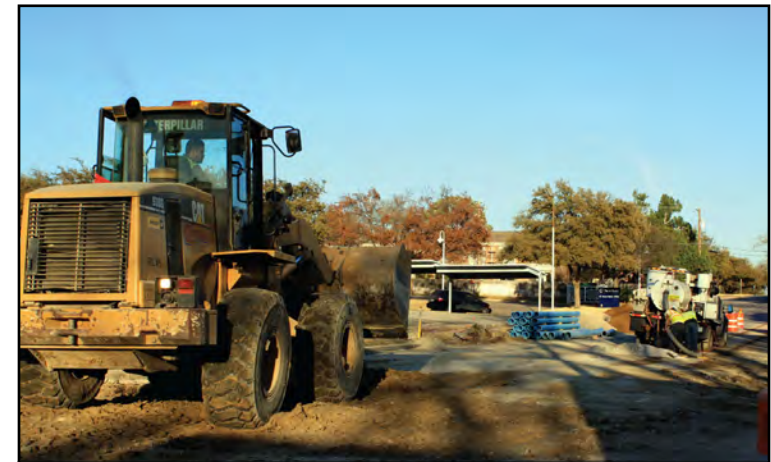
Crews breaking ground on Crestline as part of the 2007 Critical Capital Project - Part 3: Pavement Reconstruction and Water & Sanitary Sewer Replacement.
