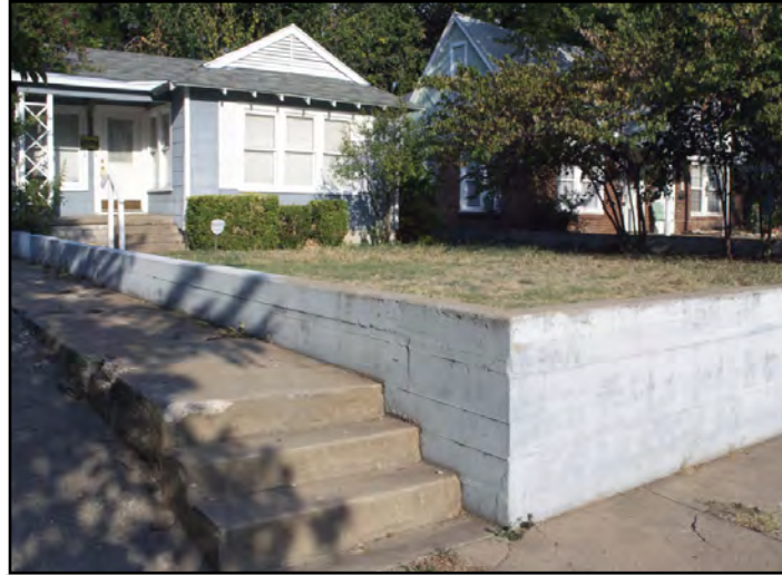
A number of property owners on Western Ave. have built concrete walls around their properties to channel overflow storm water away from their houses.
